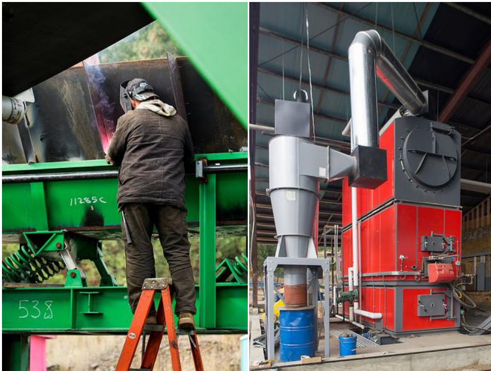
(Left) A welder puts the pieces together on the new mechanized log sorting line at Integrated Biomass Resources in Wallowa, Ore. (Right) The biomass heat system at IBR provides heat to dry firewood and electricity to the facility. Photos: Marcus Kauffman, ODF
