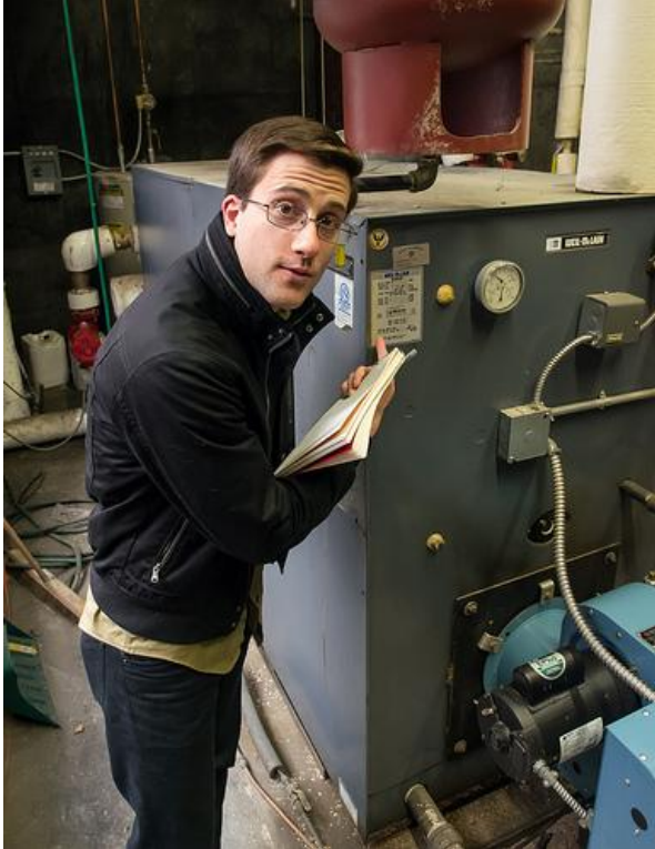
Dylan Kruse of Sustainable Northwest inspects an old oil boiler at Humboldt Elementary.
